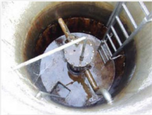
The leaking area
